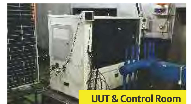
Water Chilling Facility
